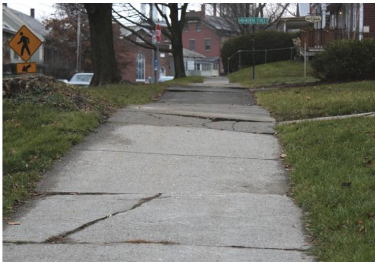
Figure 1.10: Uneven sidewalk in need of repair, on the West side of 22A, between North Street & School Street
