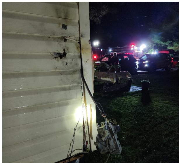
Energy meter that caught fire from Whispering Pines lightning strike in Panton, 2023
