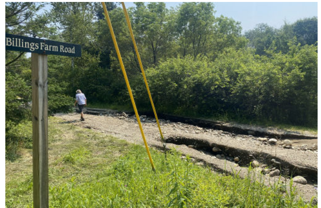
Ripton storm damage
