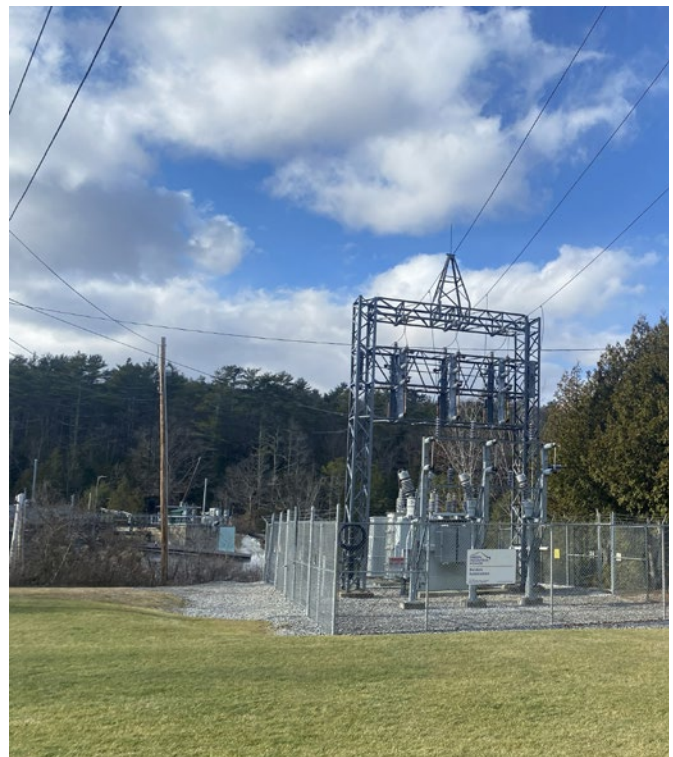
Belden Falls Substation
