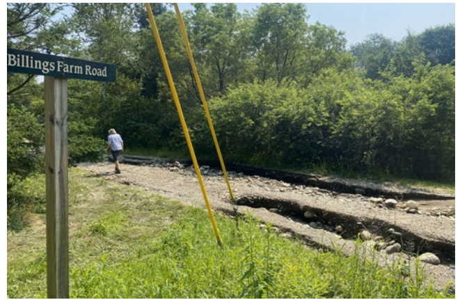
Ripton storm damage, 2024
