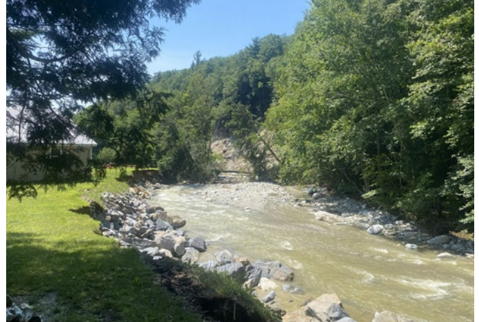
Lewis Creek erosion along Ireland Road, Bristol-Starksboro
